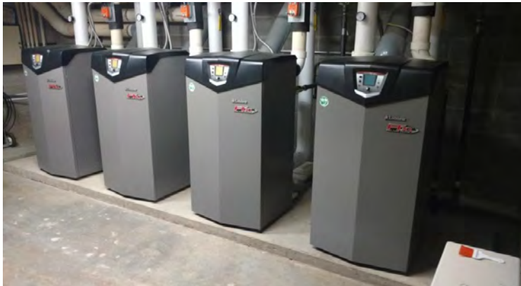
Figure: Upgraded energy efficient boilers at Marathon County Library in 2015
